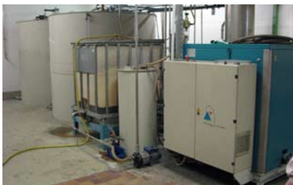
Ultrafiltration water treatment.
